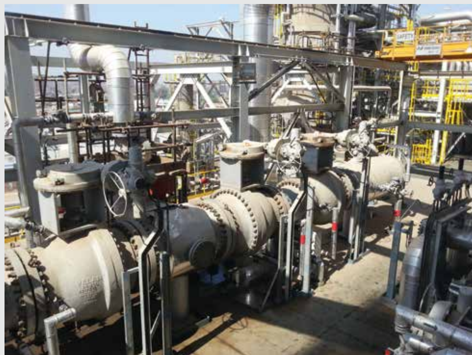
Three 36" Class 300 two-way severe service metal-seated ball valves installed at a refinery in Egypt.
