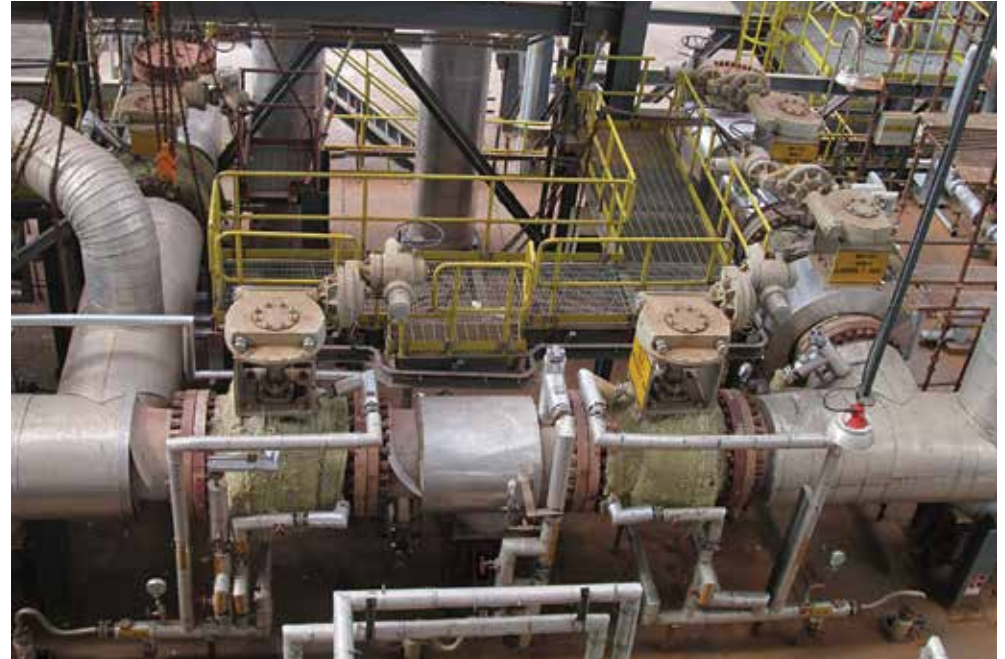
Velan coker valves in service.
