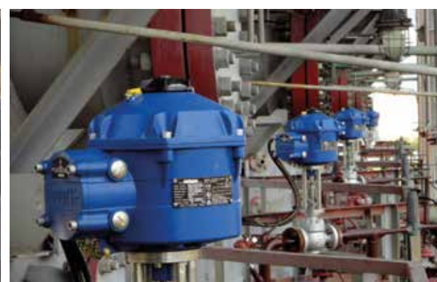
CVA range control valve actuators at an underground gas storage facility.
