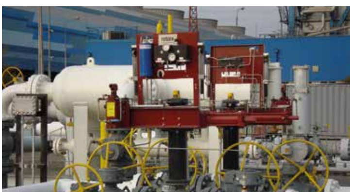
High Pressure Gas actuators at an LPG plant in Chile.
