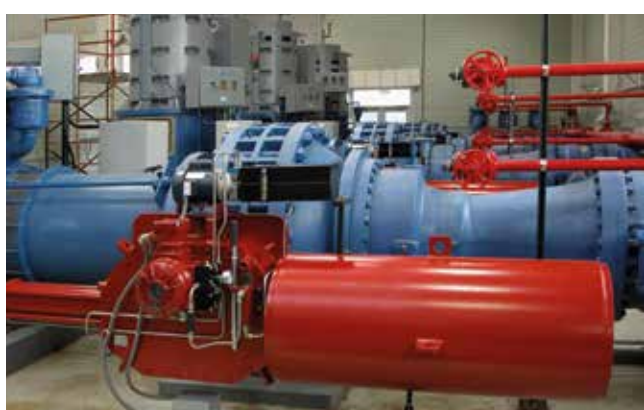
An EH range self-contained electro-hydraulic actuator at a water treatment plant.
