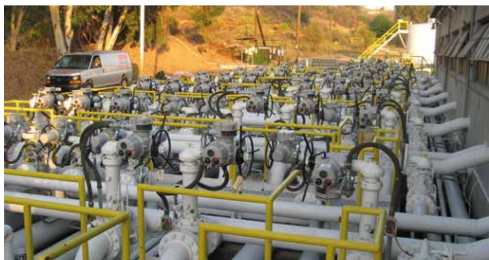
IQ actuators at a tank farm in California.
