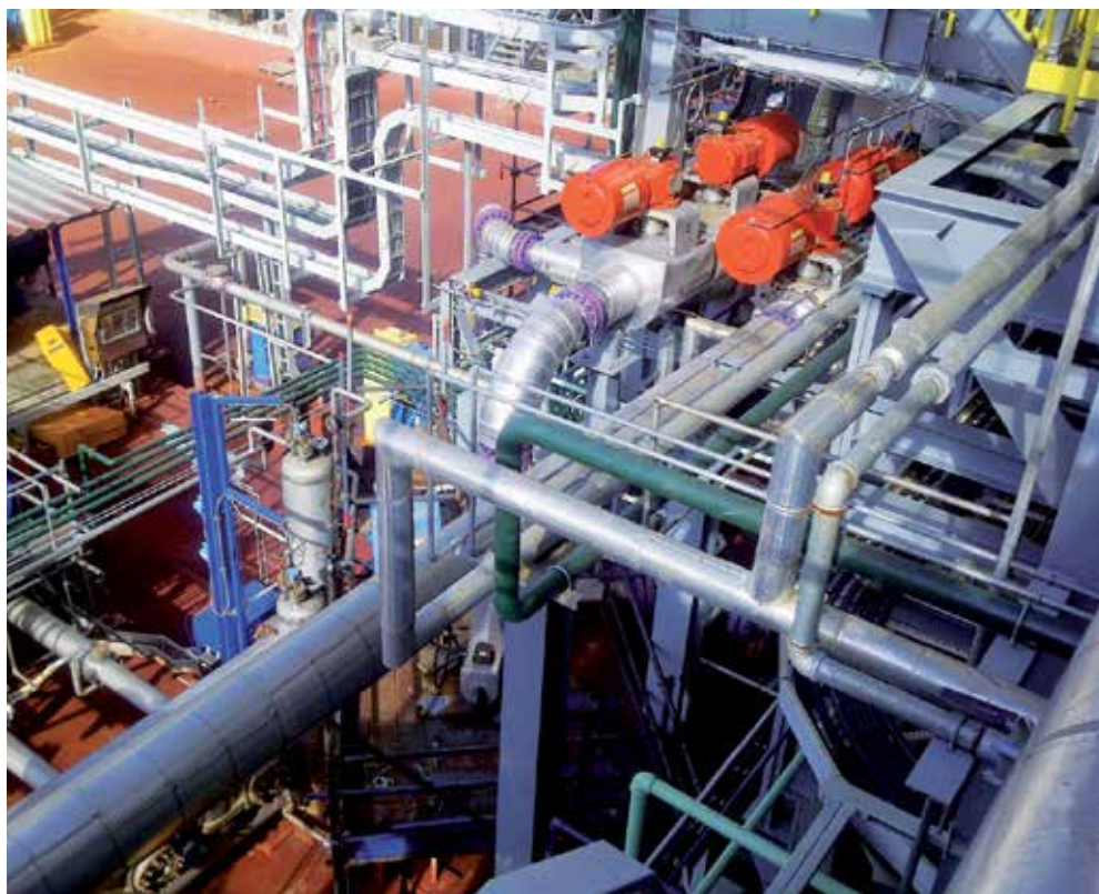
Installation of Velan valves in a nickel HPAL (High Pressure Acid Leaching) facility in Madagascar.
