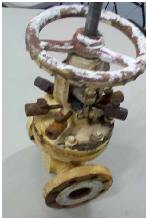
Example of valve with multiple temporary repairs.
